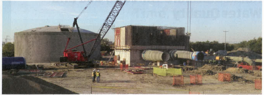
Pipeline connecting structures at the Wylie Water Treatment Plant include a 240-million-gallon balancing reservoir, five ground storage tanks, new metering vaults, blending structures (pictured), chemical feed systems, and electrical, SCADA and security system upgrades.
